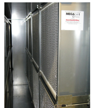
MEGAcel® I filters installed in Cancer Treatment Centers of America®
